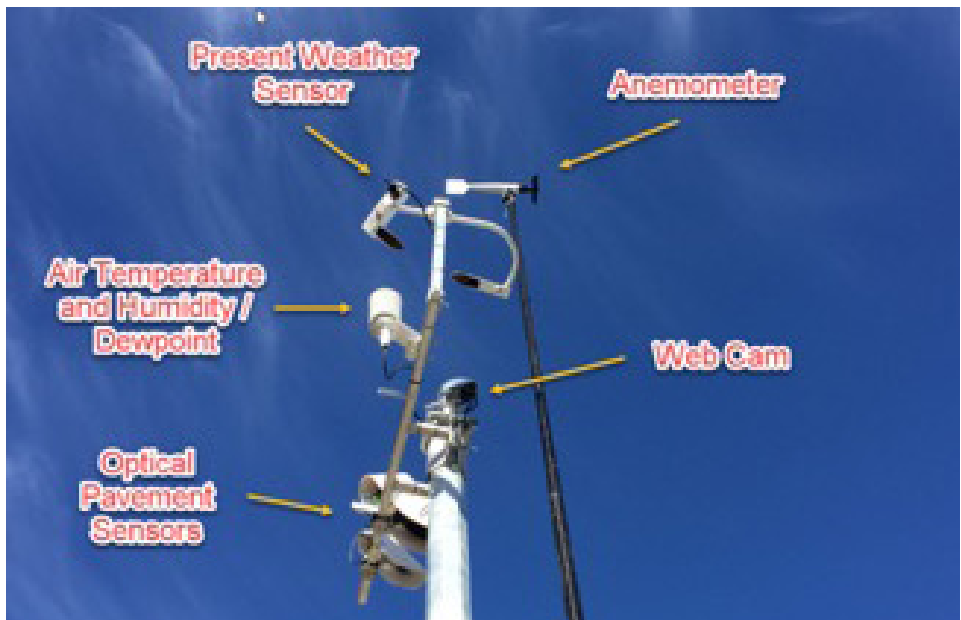
Road Weather Station Sensors
