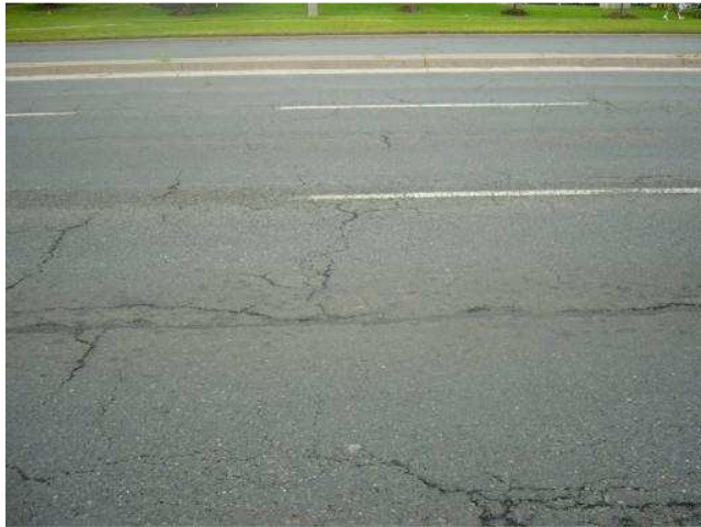
Figure 3 - Section of Highway 7 showing typical distresses; transverse, longitudinal and pavement edge cracks, ravelling and rutting.
