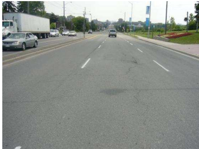
Figure 1 – Overview of Yonge Street looking at the southbound lanes. Note the transverse cracks and the mid lane crack in Lane 2.
