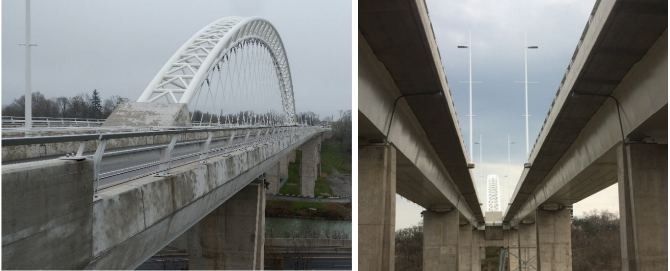
Figure 3 – Burgoyne Bridge Exterior Edge (Left) and Interior Gap (Right)
