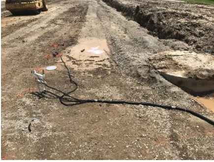
a. Overall view of installed sensors
