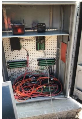
e. Data station
