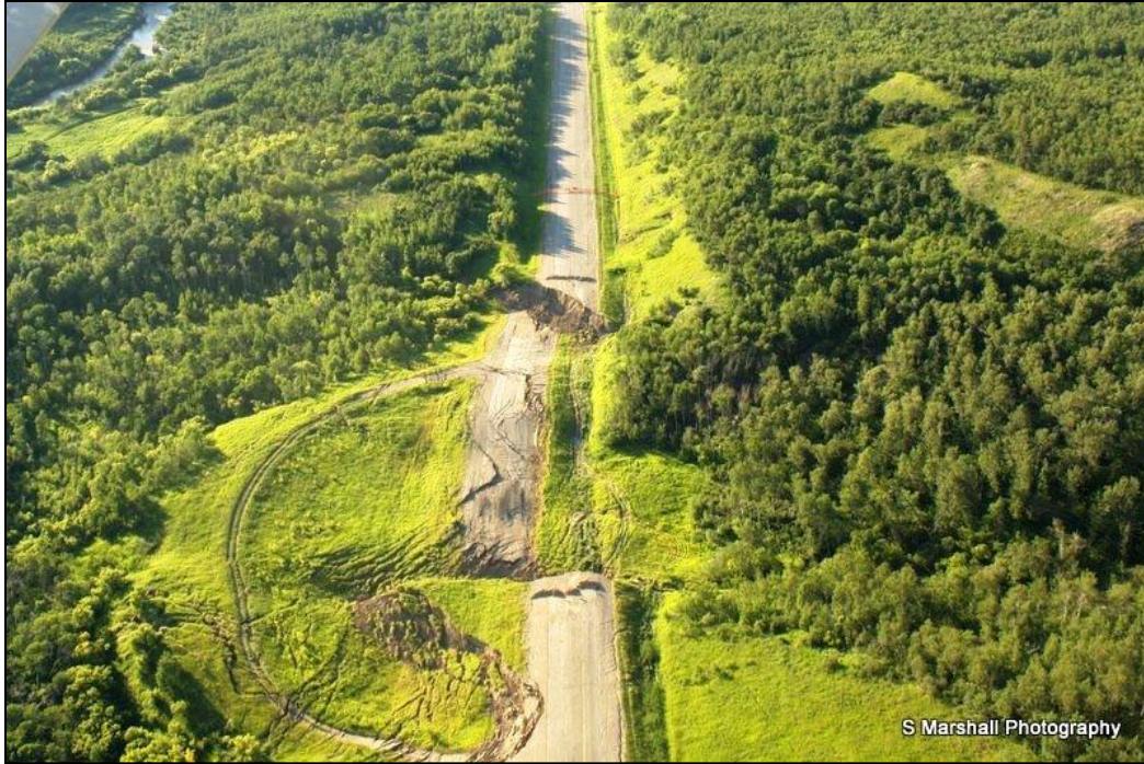
Photo 1: Aerial view of PTH 83 Shell River Landslide July 2012 (courtesy of Shelia Marshall)
