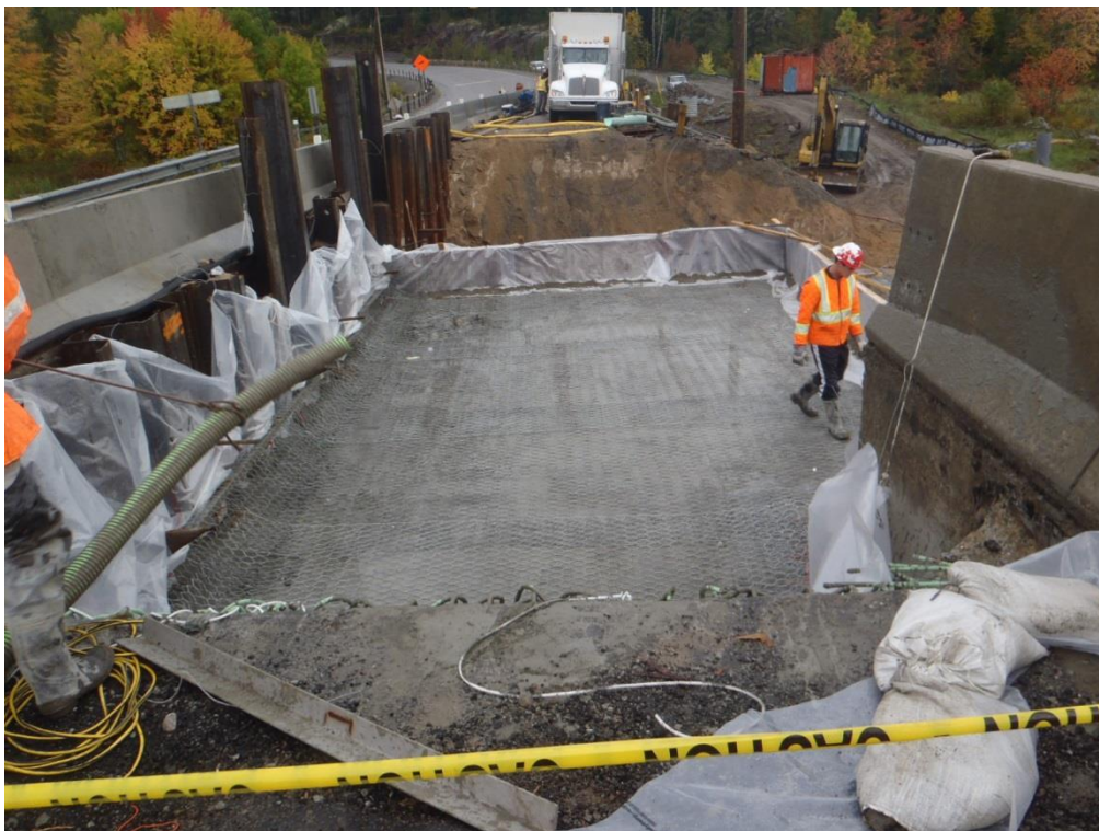
Photo 4 – Staged Construction of Embankment. Exposed subsoil of slag fill seen on the background
