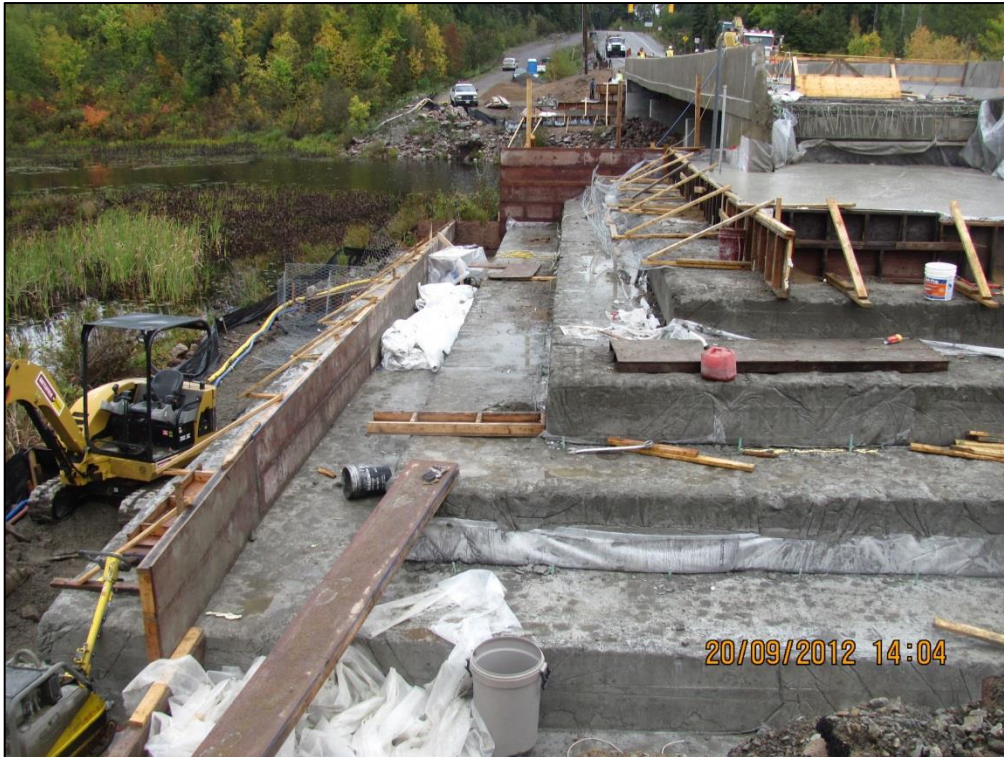
Photo 1 – Construction of southern embankment. Lighter formwork was used due to the lower unit weight of cellular concrete. Wire mesh was used as part of tie-down system using gabion blocks.
