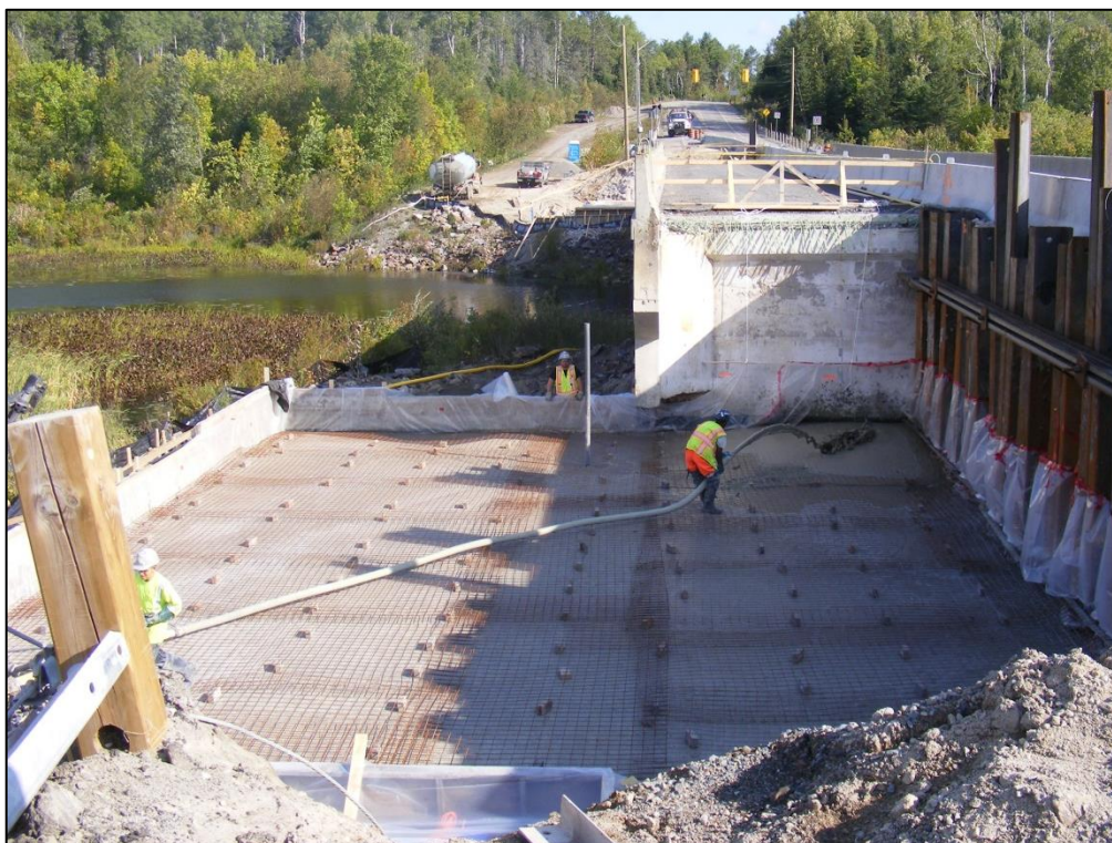
Photo 2 – Placement of cellular concrete. Plastic sheets were used to make the forms impermeable and secondary containment was installed to guard against unplanned concrete discharge or spills
