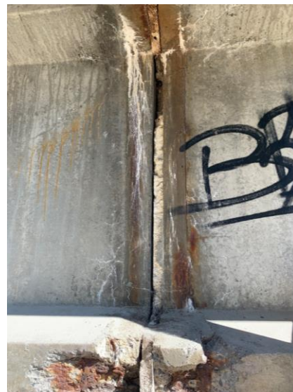
Figure 8 - Girder ends with spalling and corroded strands
