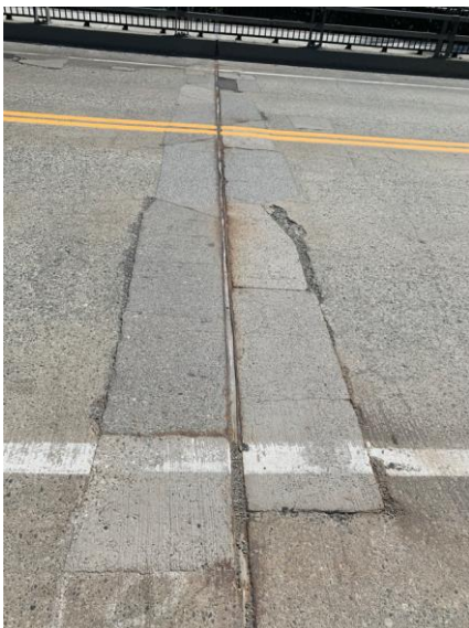
Figure 7 - Deteriorated deck joint and concrete
