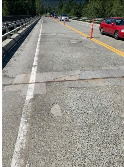
(b) Surface patches around deck joints
