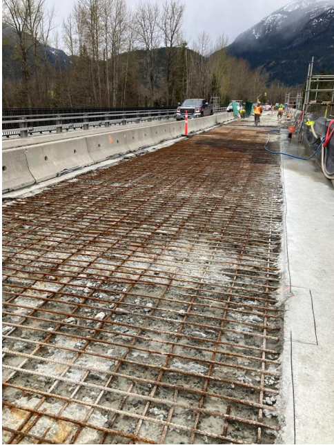
Figure 14 - Exposed rebar after partial deck removal
