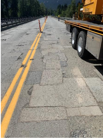
Figure 3 – (a) Deteriorated surface with patches
