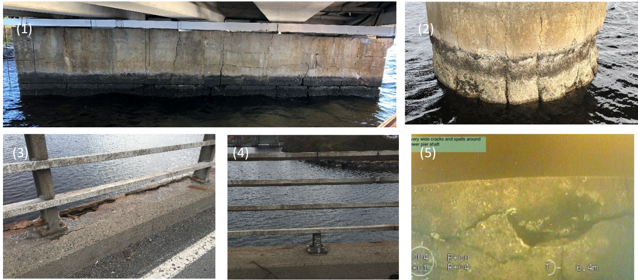
Figure 5. Condition of existing structure (1) wide pattern cracking in the south abutment; (2) severe scaling at the water line and wide vertical cracks in the upper pier shafts; (3) Exposed rebar in curbs and overhangs; (4) broken and missing rail posts; (5) very wide cracks and delamination of the lower pier shafts
