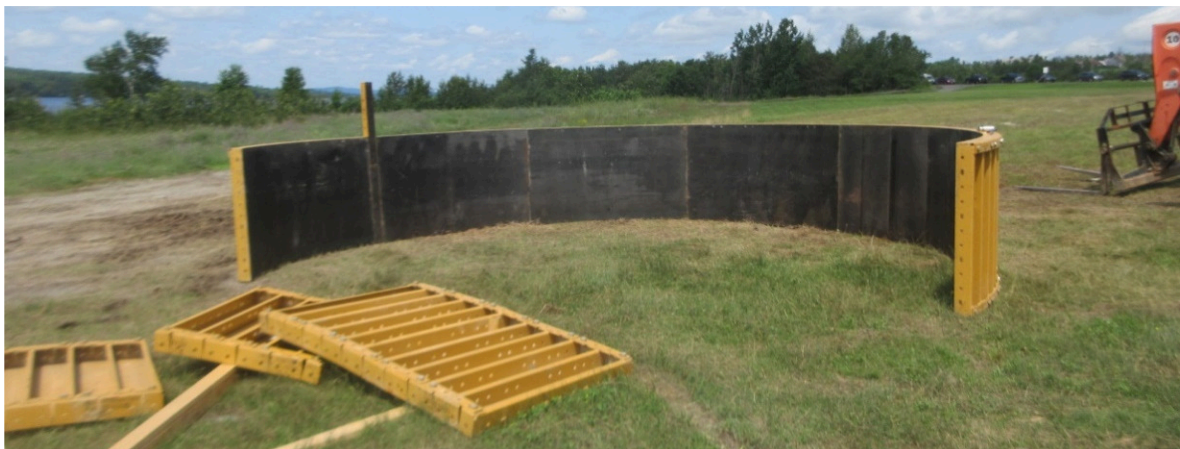
Figure 16. Dry fit of circular EFCO form on grade before lowering segments and installing form on lower pier shafts underwater for eventual tremie concrete placement
