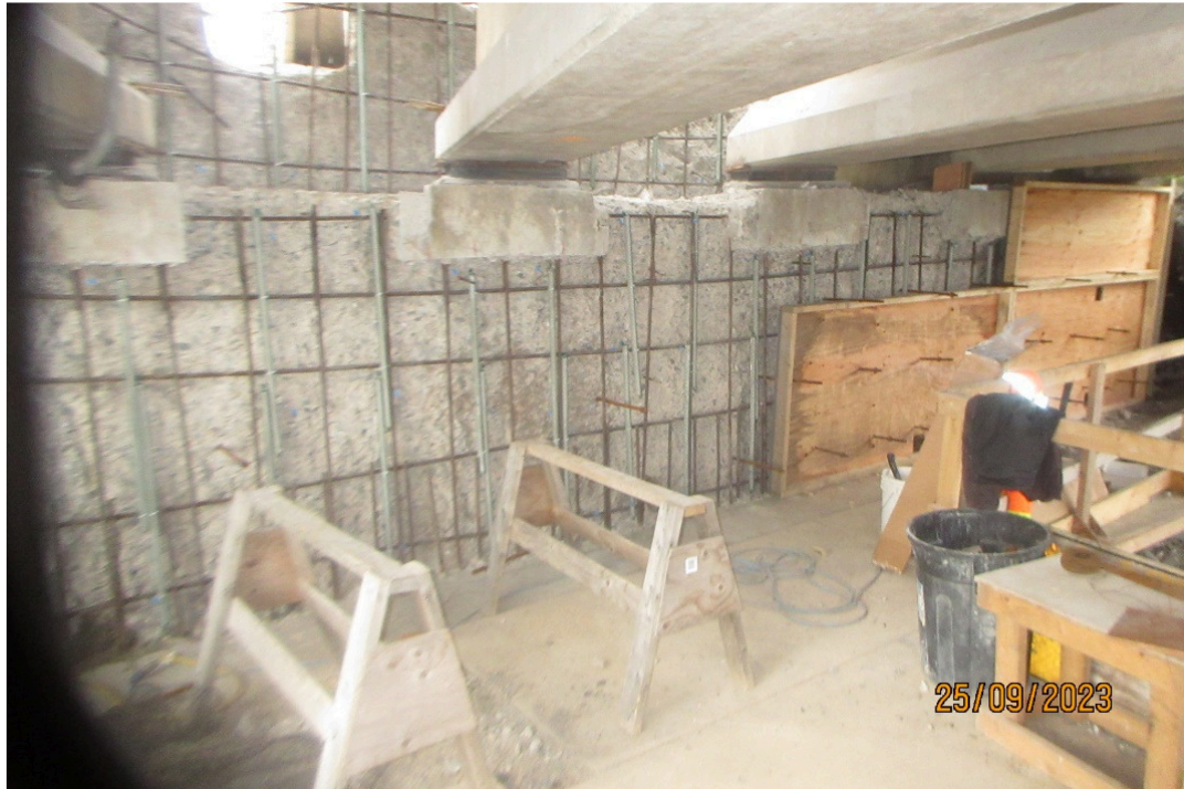
Figure 17. North Abutment breastwall has been reconstructed incorporating a distributed anode system. Bearing replacement will be completed later.
