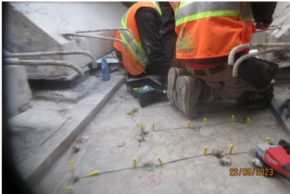
Figure 18. Hybrid Fusion galvanic anodes being installed into the top surfaces of the pier hammerheads by Vector Corrosion Technologies.
