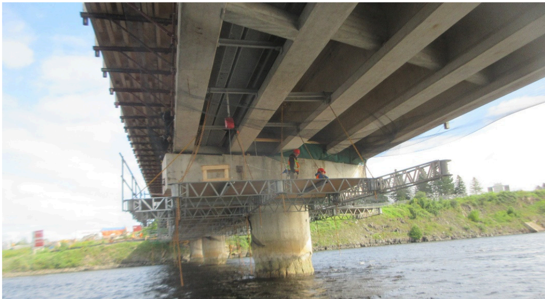
Figure 14. Suspended scaffolding erected under bridge for pier encapsulation and bearing replacement work.
