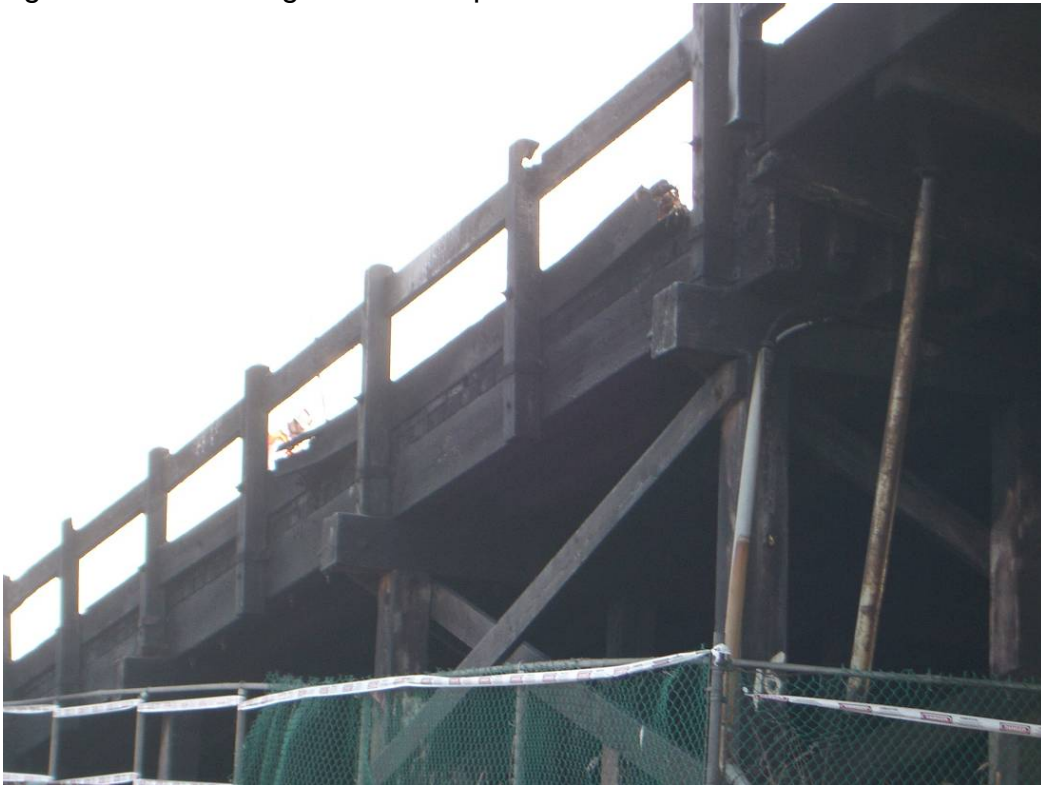
Figure 3. Close up of Fire Damage
