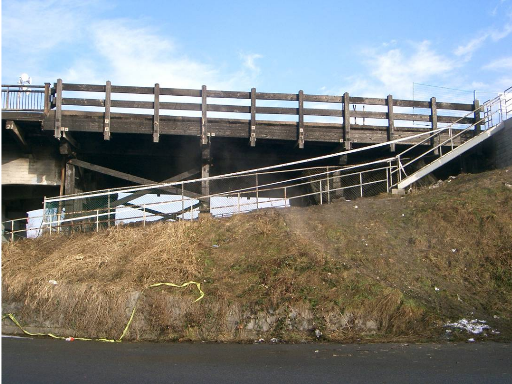
Figure 2. Fire Damaged Timber Spans
