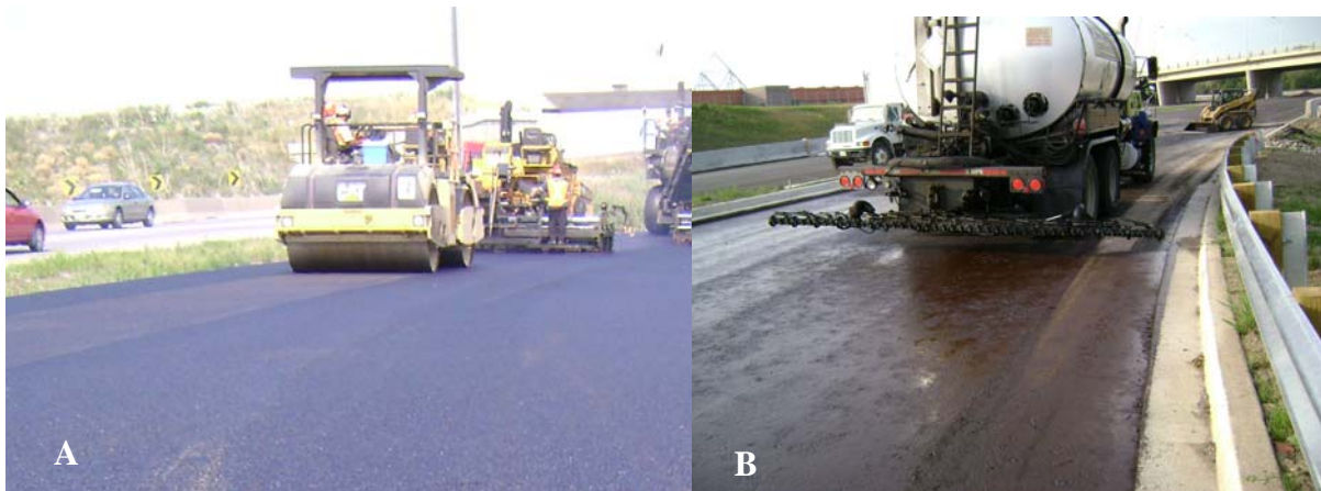
Photograph 8. In order to achieve compaction of the SMA layer, the rollers were kept very close to the paver screed (A). Application of tack coat on the surface of the Superpave 25 layer (B).
