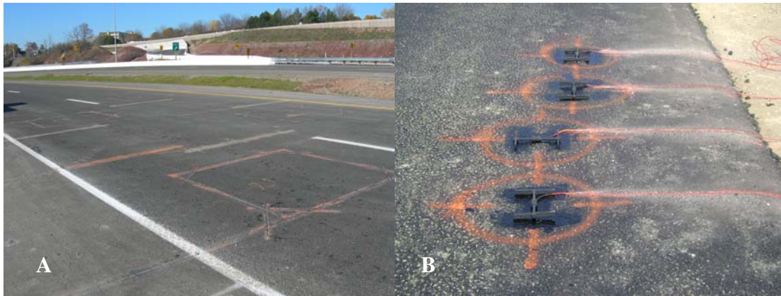
Photograph 10. Traffic loops and Weigh in Motion sensors installed in the pavement (A) and the tensile asphalt gauges on the top of the Superpave 19 layer ready to be covered with the SMA surface course layer (B).
