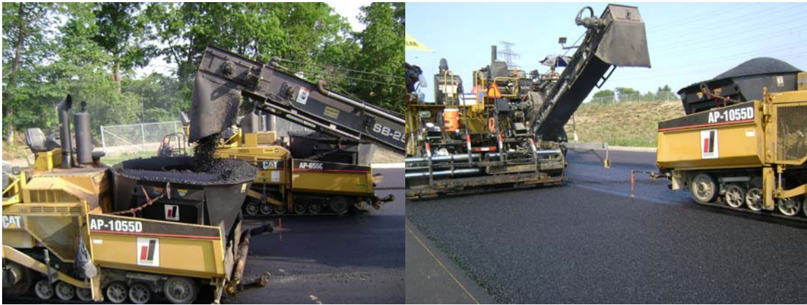
Photograph 3. Echelon paving of the SMA surface course using a Material Transfer Vehicle (MTV).
