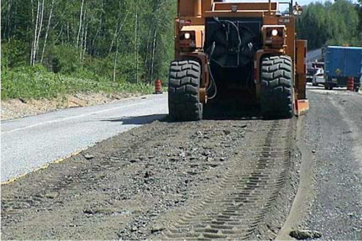
Figure 5. Pavement with “alligator” cracks after pulverization
