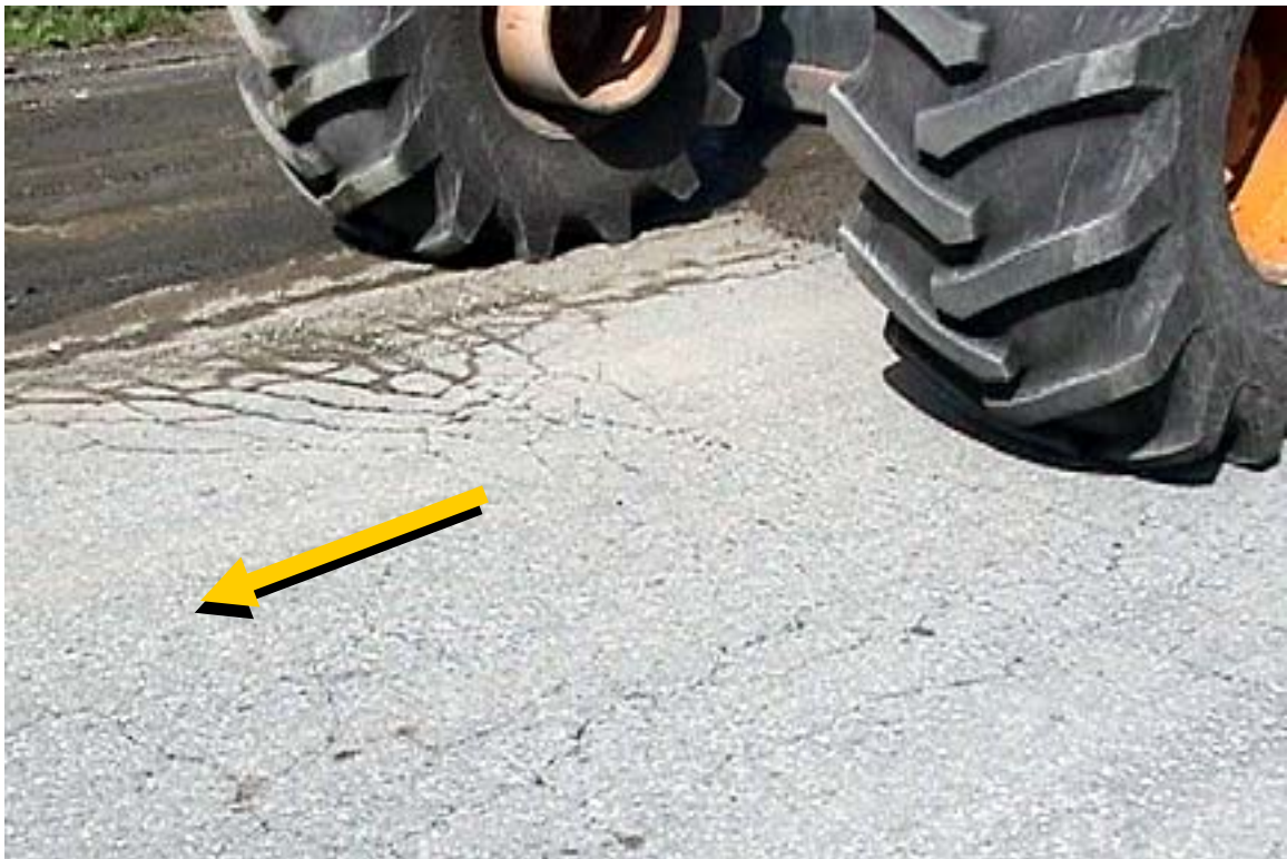
Figure 4 "Alligator" cracks in pavement prior to pulverizing (direction of travel shown)
