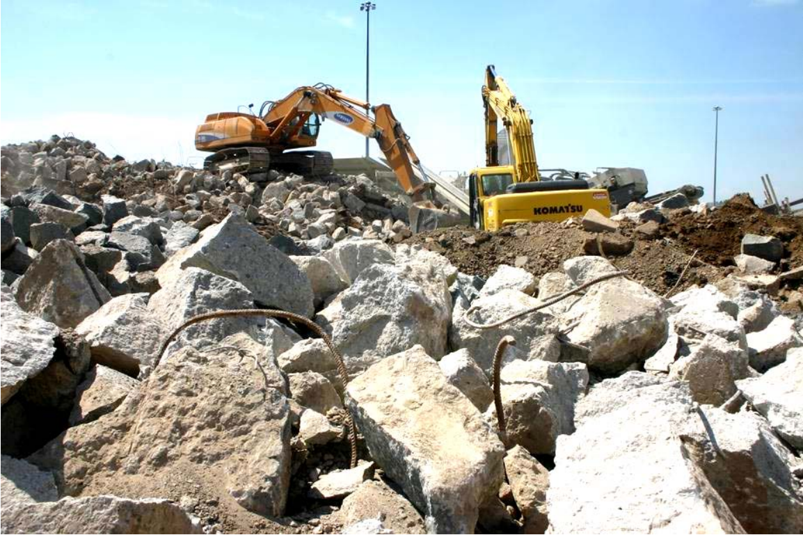
Figure 1. Reclaimed concrete material from an MTO bridge structure being prepared for crushing into aggregate for granular base
