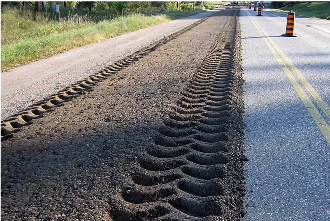
Figure 2. Full depth reclamation product - pulverised pavement and underlying granular material blended to produce new aggregate base material
