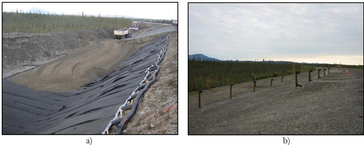
Figure 9: a) Backfilling over geocomposite on slope heat drain section. b) View of finished heat drains with insulation section.
