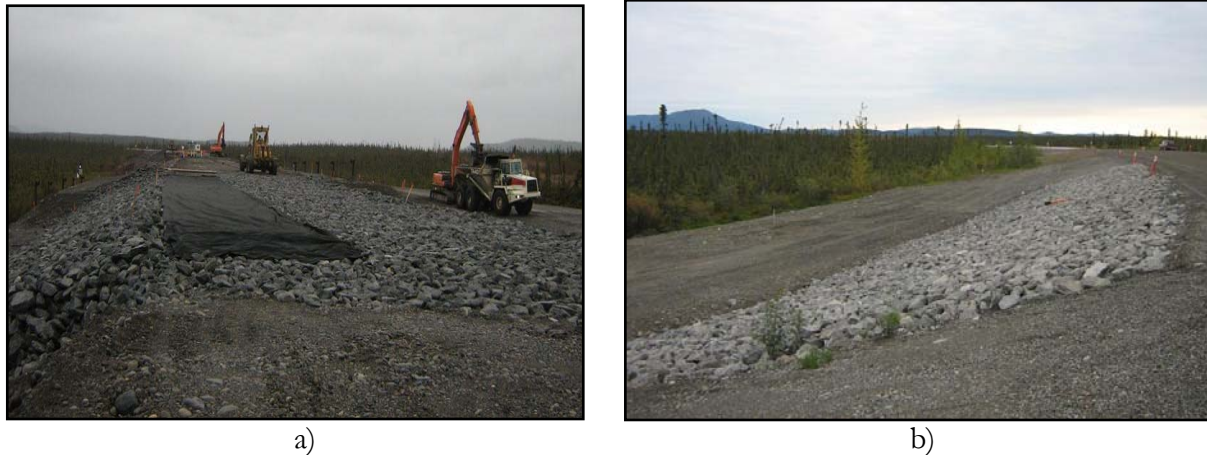
Figure 5: a) Full ACE embankment built; placing geotextile prior to base course. b) Finished uncovered ACE slopes section.
