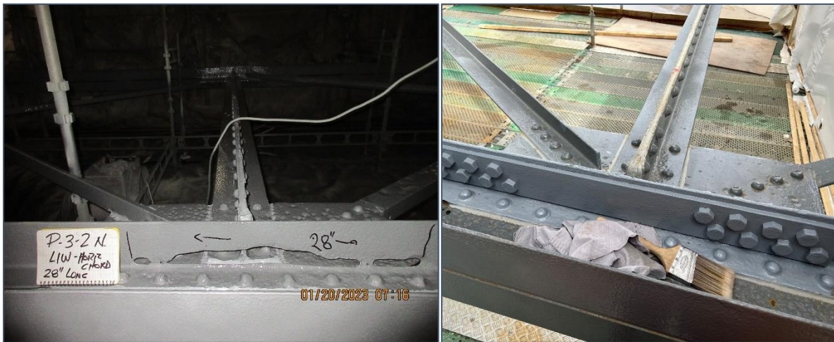
Figure 22: Large Holes in Primary Tension Member (left) and Completed Typical Repair (right)
