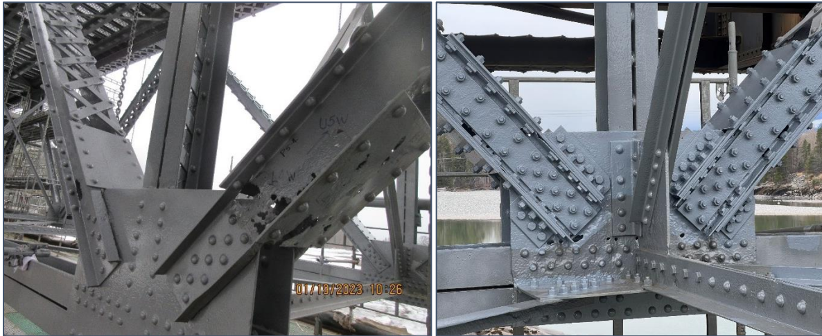
Figure 21: Large Holes in Primary Diagonal Members (left) and Completed Repairs (right)
