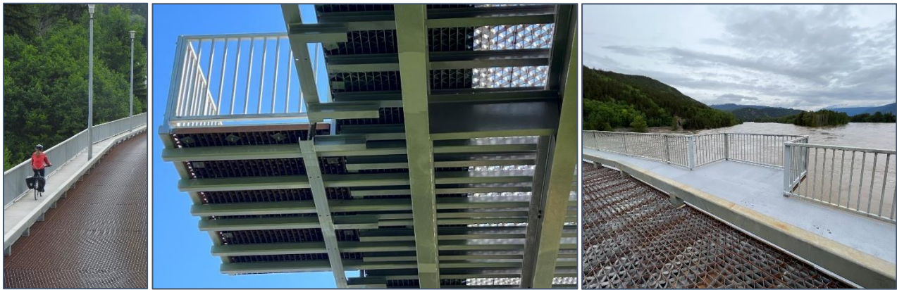
Figure 12: Sidewalk Refuge Bays with Existing Narrow Sidewalk (left), Support Beams (centre) and Finished Bay (right)
