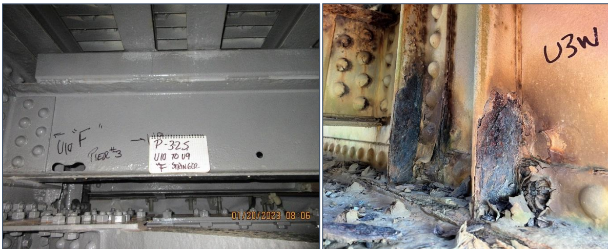
Figure 23: Post-Blast Clean Damage to Stringer (left) and Pre-Blast Clean Floor Beam Bearing Stiffeners (right)
