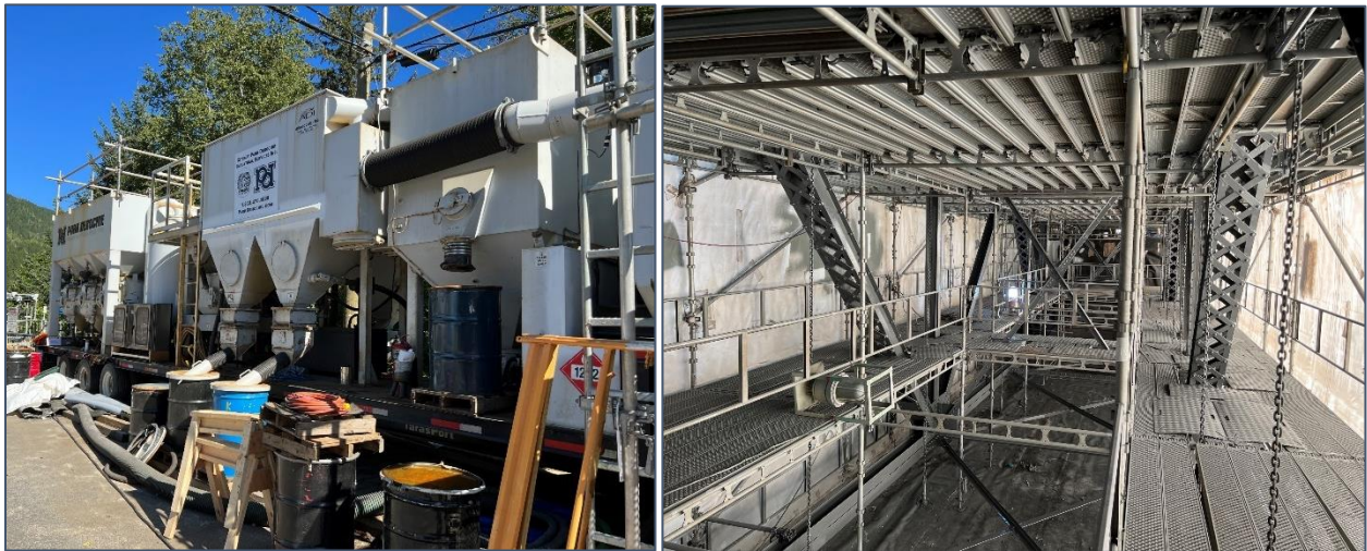
Figure 18: Steel Shot Blast Recycling Equipment (left) and Inside a Coatings Enclosure Following Top Coat Application (right)
