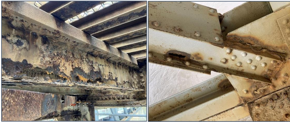
Figure 9: Examples of Severe Corrosion in Deck Stringer (left) and Truss Diagonal (right)
