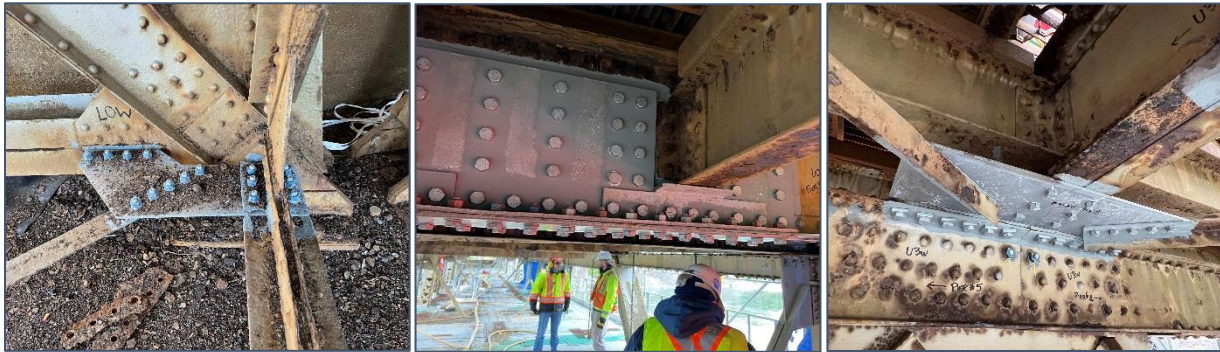
Figure 11: Typical Repairs at Lower Gusset (left), Floor Beam (centre) and Upper Gusset (right)
