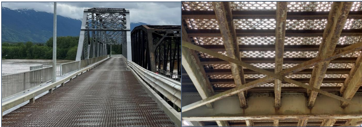
Figure 5: 2001 Steel Deck System from Above (left) and Below (right). Decking Supported on Existing Stringers and Floor Beams
