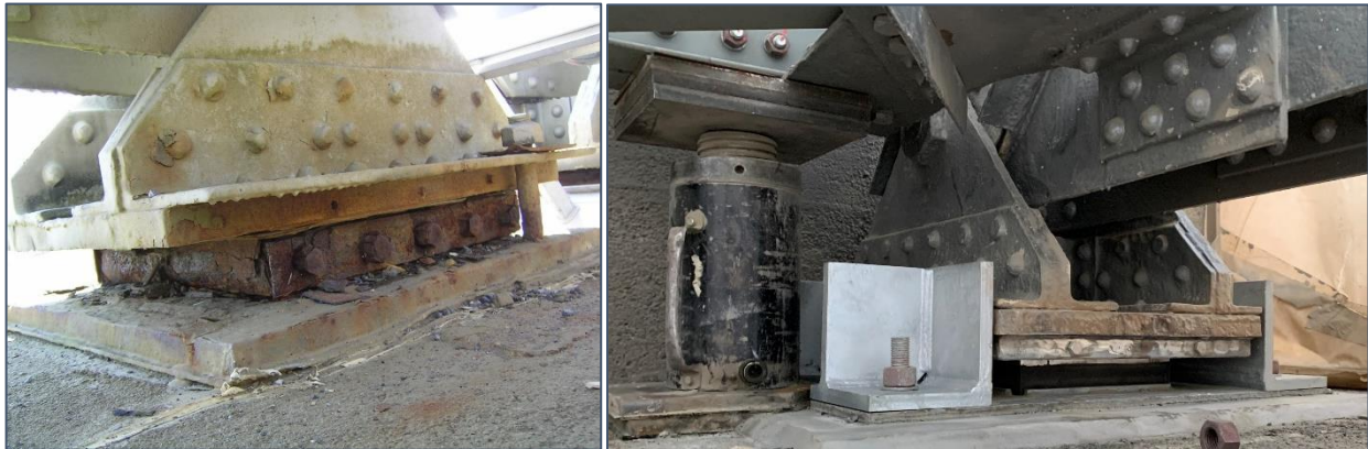
Figure 10: Existing (Seized) Roller Bearings (left) and New Sliding Elastomeric Bearings with Lateral Restraint (right)
