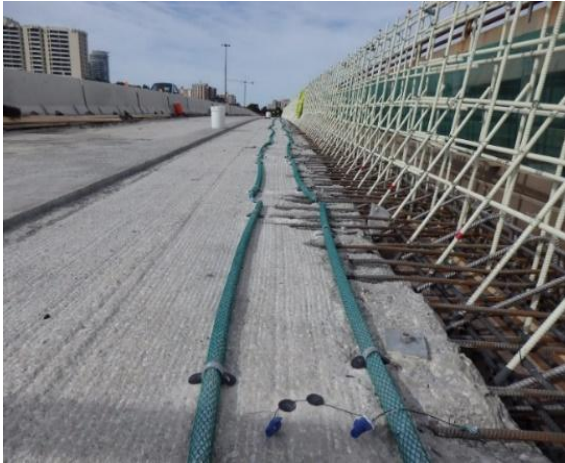
Figure 7. Distributed Anodes installed at the edge of existing deck for the parapet wall replacement to prevent corrosion from initiating, Toronto, Canada
