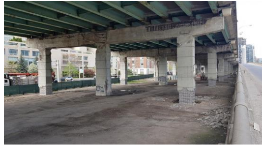
Figure 1. Pier Corrosion Due to Chloride from Leaking Joints and Roadside Splash
