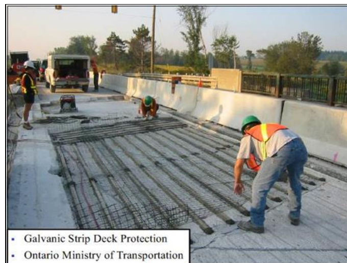
Figure 10. First Trial of DAS Anodes in Bridge Deck Overlay, Ontario, Canada, in 2003
