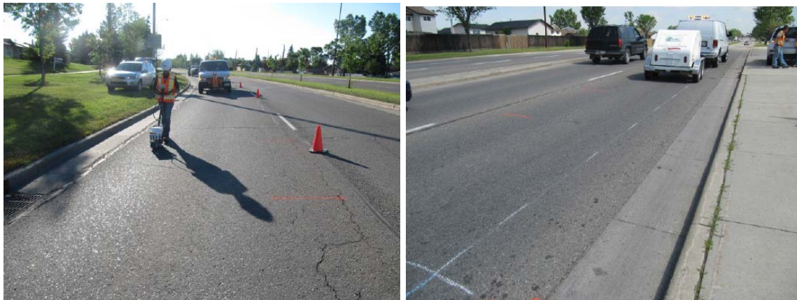
Figure 9: SurPRO profile and GPR surveys and FWD testing on one of the pavement sections included in the City of Calgary PDF study.
