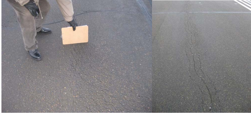
Figure 16: Severe asphalt shoving and cracking on Runway 12-30 at Edmonton International Airport observed in 2013
