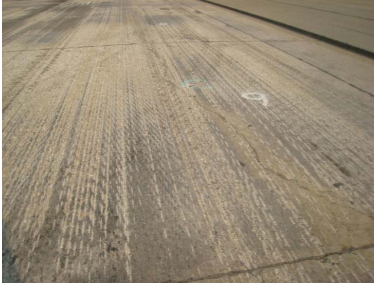
Figure 19: Stitched concrete slab before placement of asphalt overlay on Runway 12-30 at Edmonton International Airport in 2013.
